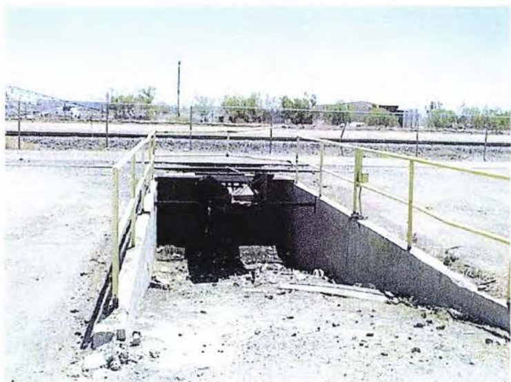
Photograph 9 - View of the railroad siding and railroad car unloading conveyor on the northeastern portion of the subject site. The eastern adjoining concrete plant is seen in the background.
