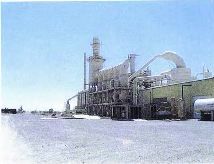
Photograph 3 - View of industrial equipment attached to the northeastern portion of the main building.
