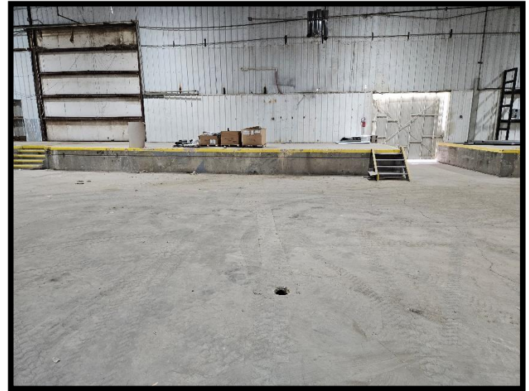
26-Floor drain with saw-cut leading E towards pipe at base of E wall of main building
