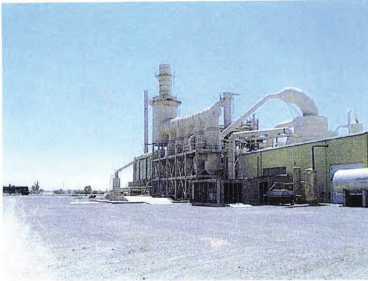
Photograph 3 - View of industrial equipment attached to the northeastern portion of the main building.
