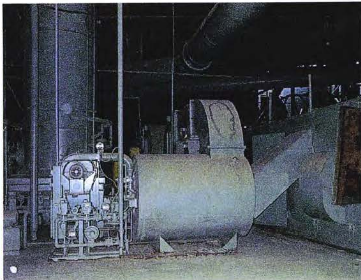
Photograph 8 - View of industrial equipment inside the main building.
