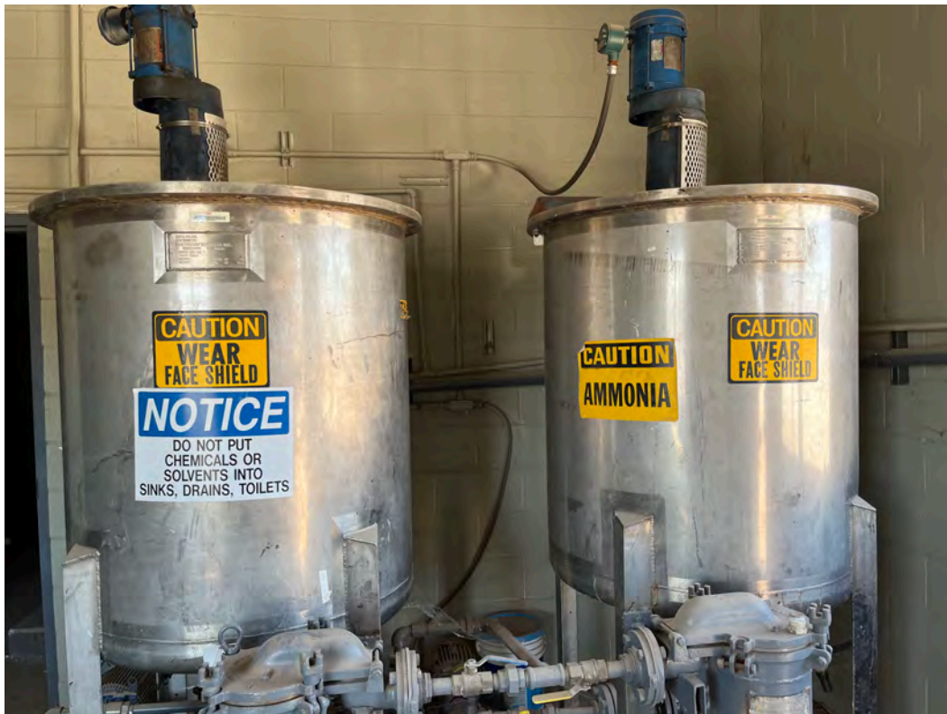
Photo 22: Equipment in small manufacturing building.
