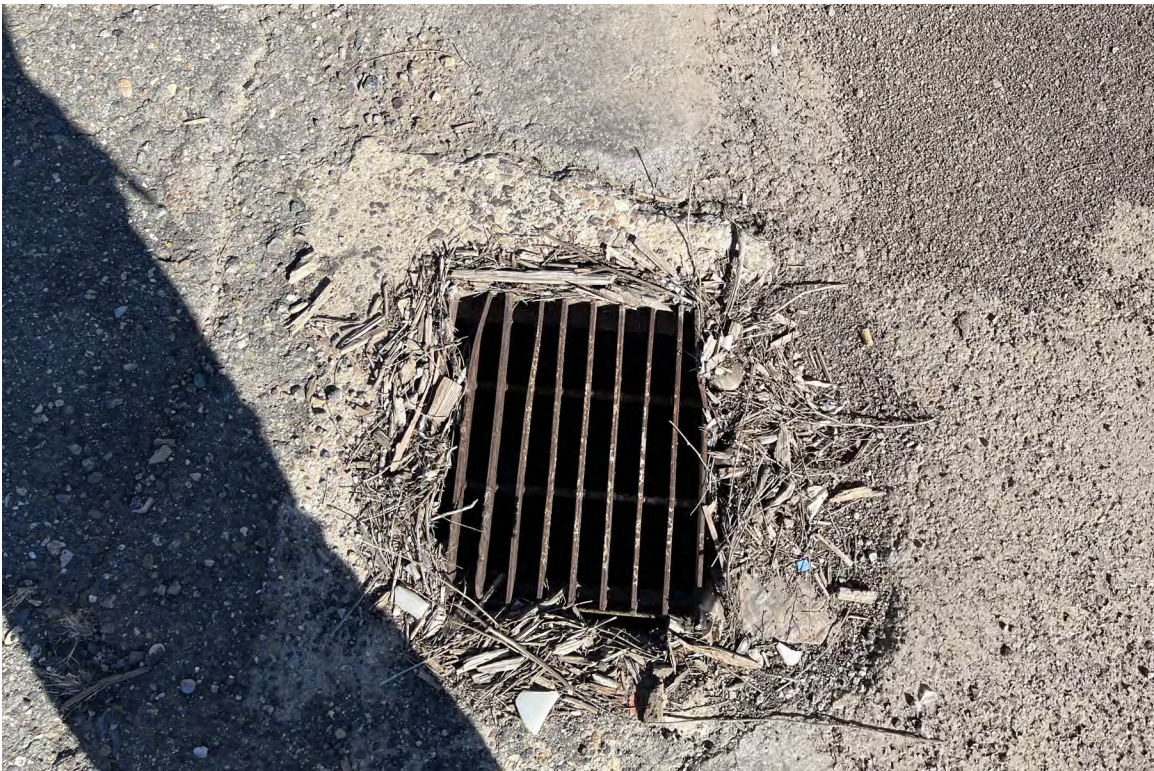
Photo 4: Drain inlet that discharges into Loading Dock.
