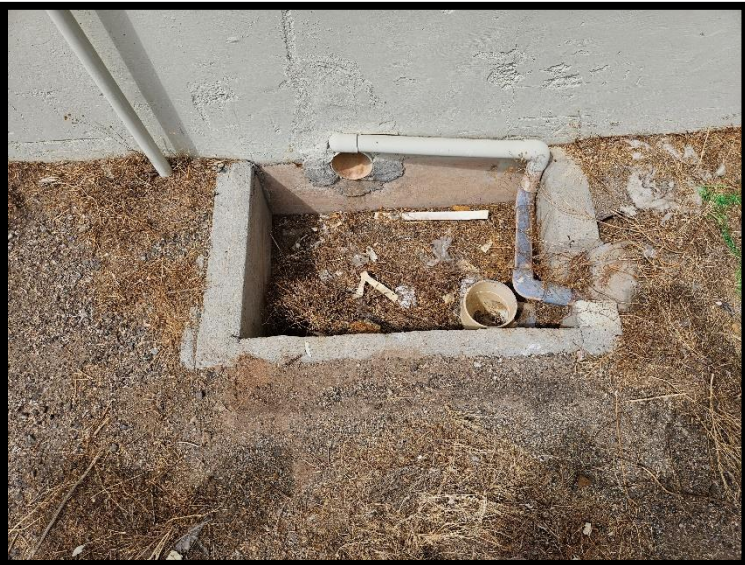
23-Drain sump from inside main building along S quarter of E side of main building
