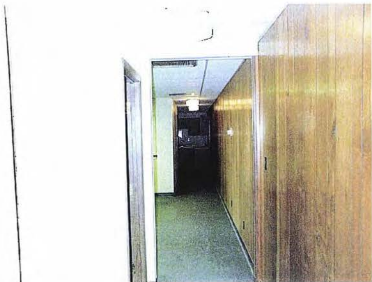
Photograph 7 - Interior view of the hallway and office space in the western portion of the main building.
