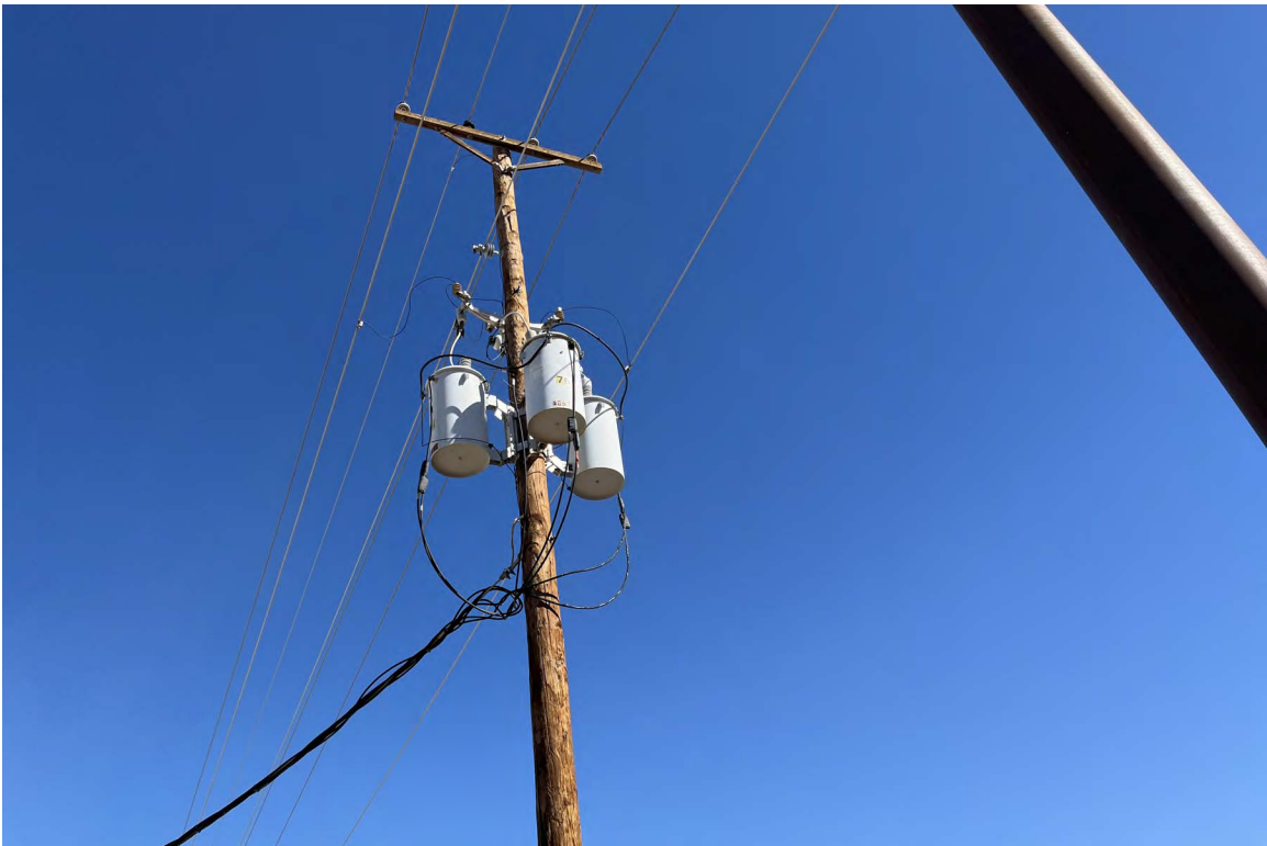
Photo 14: Pole mounted transformers by warehouse building.
