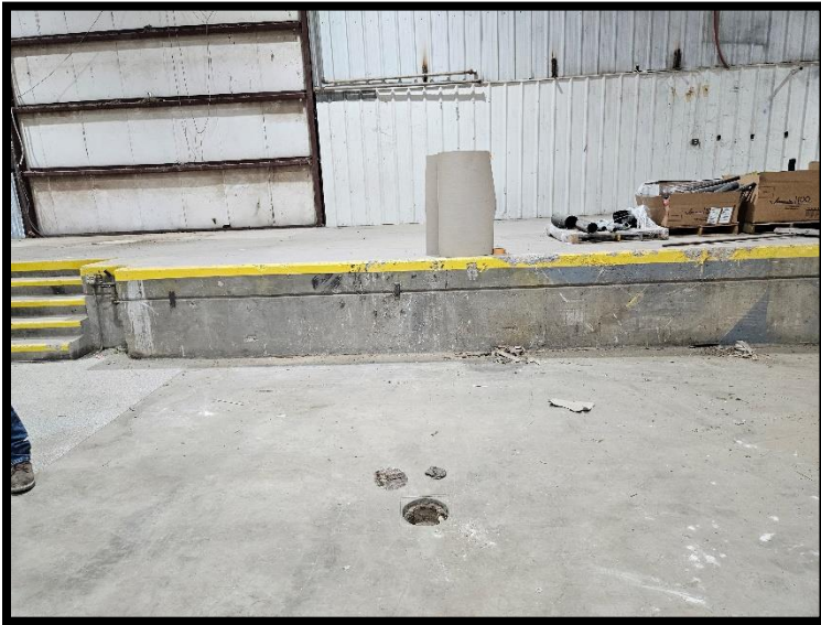
25-Drain that drains to sump (photo 23) along E side of main building
